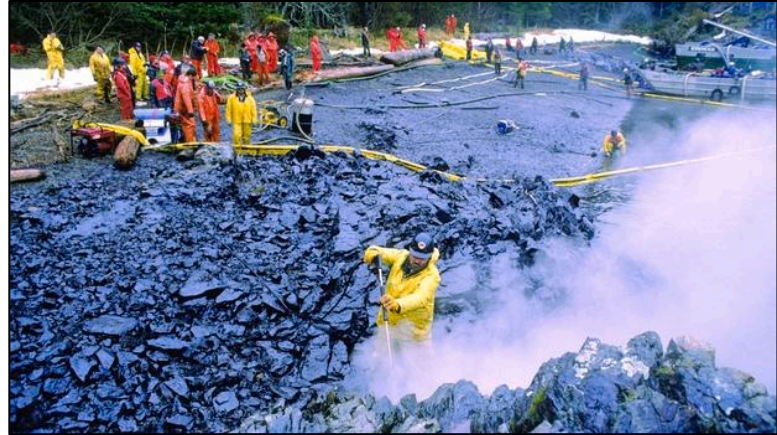
Figure 9 – Cleanup of Oil-Soaked Beach at Eleanor Island, Alaska April 16, 1989 (Source: McClatchy Newspapers)
